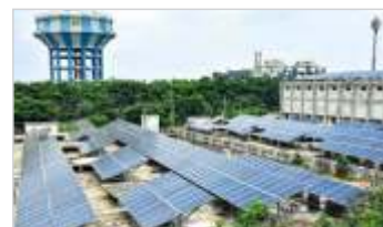
1000KWp Surat Municipal Corporation Gujarat
