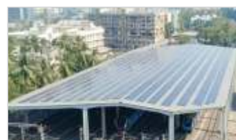
1200KWp Reliance Metro Mumbai
