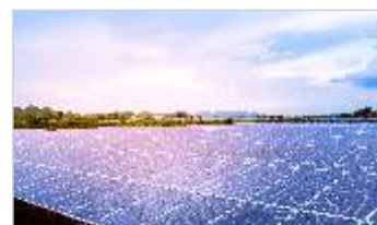
40 MWhr Continuum Green Energy Gujarat (Under Commissioning) BATTERY STORAGE EPC PROJECT
