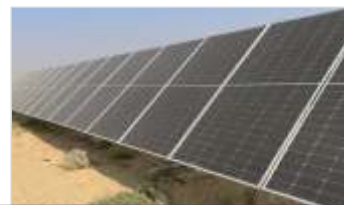
412.5MWp Acciona ISTS Solar Plant Bikaner, Rajasthan (Under Commissioning)
