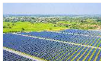
980MWp Greenco Solar Power Project Kurnool, Andhra Pradesh (Under Commissioning)
