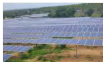
44MWp Hero Future Energies Telangana
