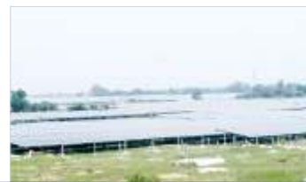
100MWp Waareep Solar Pvt. Ltd. Madhya Pradesh & Andhra Pradesh
