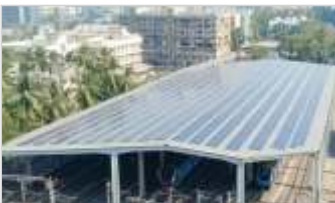
1200KWp Reliance Metro Mumbai
