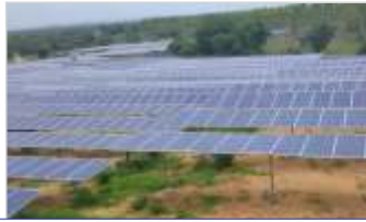
44MWp Hero Future Energies Telangana
