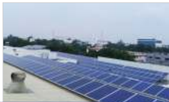
450KWp Orbit Bearings Gujarat
