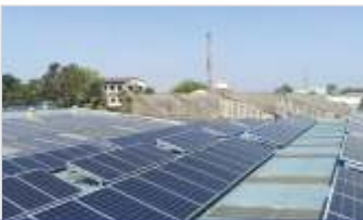
700KWp MSL Driveline System Ltd. Maharashtra
