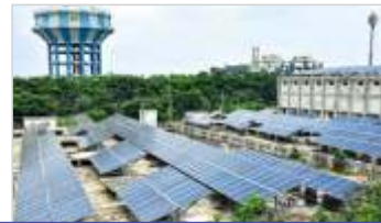
1000KWp Surat Municipal Corporation Gujarat
