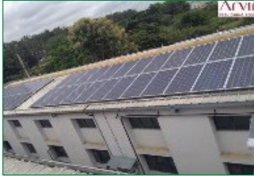
Company : ARVIND MILLS Capacity : 800 kWp
