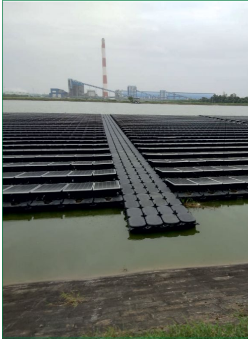
1 MW NTPC, KAWAS, SURAT
